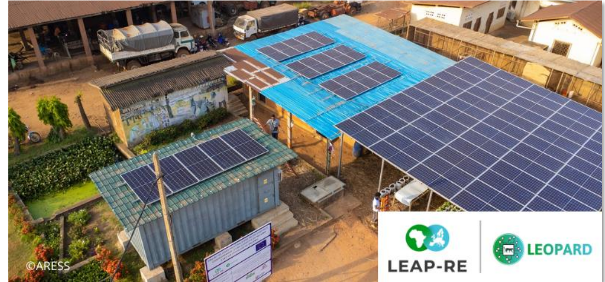
LEOPARD demonstrator installed on the Centre Songhaï campus in Benin (2022)
